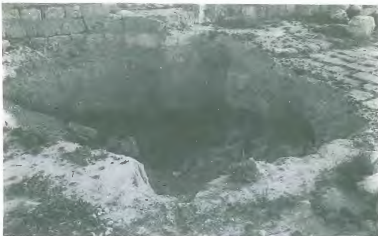
a. Water destructions in Abu Mina, a collapsed underground cistern below the south wall of the sepulchral church (Grufkirche)
